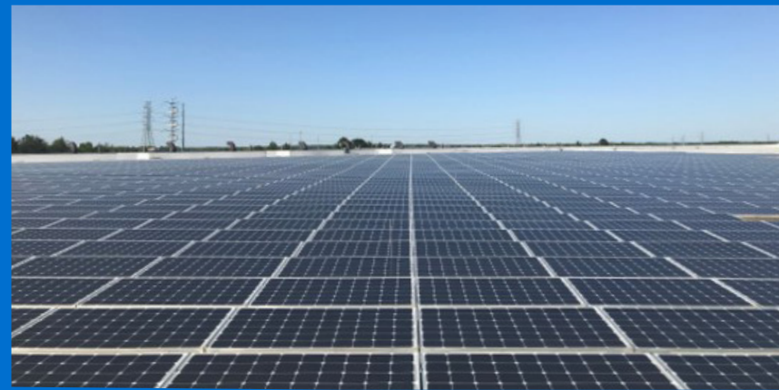
The rooftop solar at our North Carolina data center
