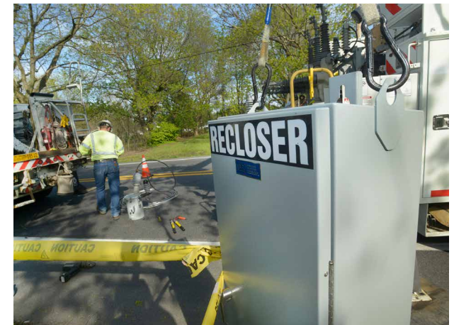
Exelon is using many technologies to make our systems more resilient, such as “reclosers” that automatically reset circuits after an interruption.
