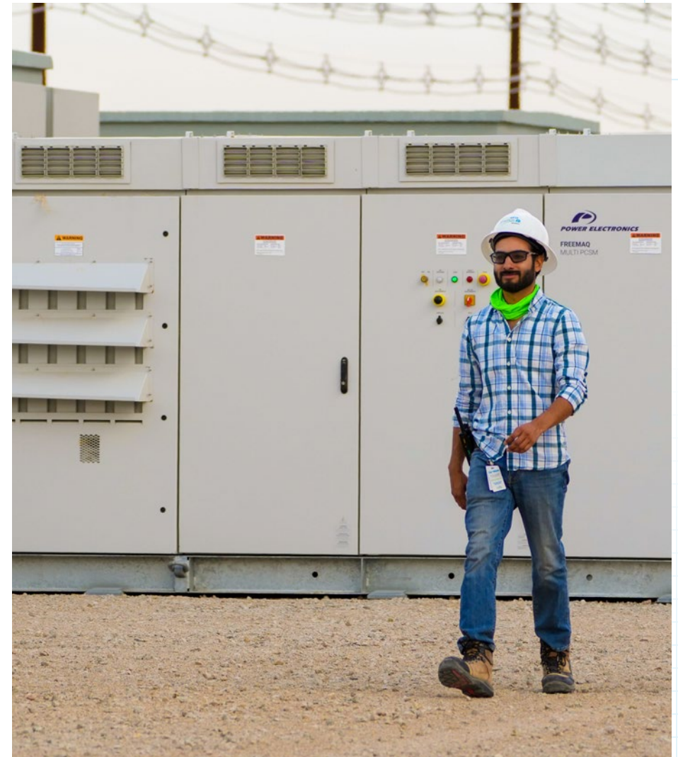
Employee Francisco Castellanos checks on the battery energy storage facilities Blythe and McCoy Energy Centers in Blythe, Calif.
