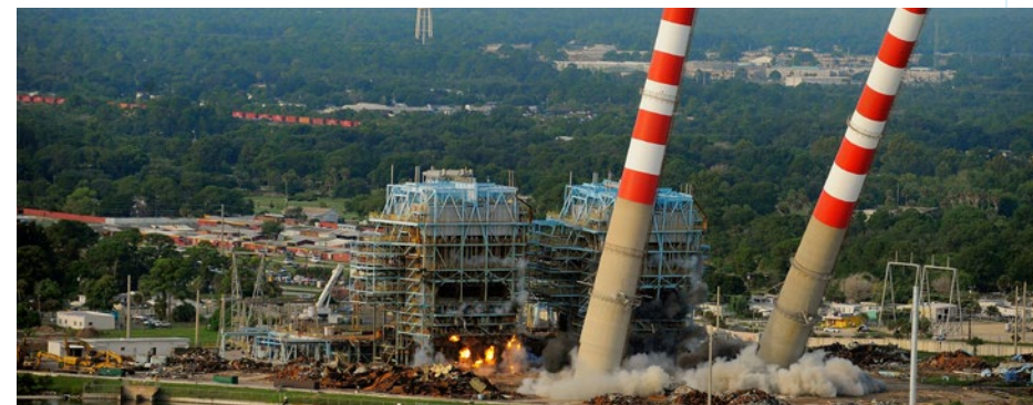
The distinct red and white stacks of FPL's Cape Canaveral Power Plant in Florida are demolished to make way for a more modern, efficient, less-carbon emitting facility to serve Florida customers.
