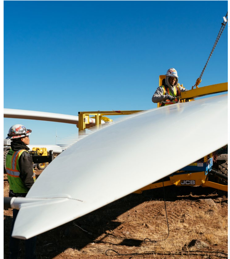
Crew members team up to install new wind generating equipment during construction of the Borderlands Wind Energy Center in Quemado, N.M.
