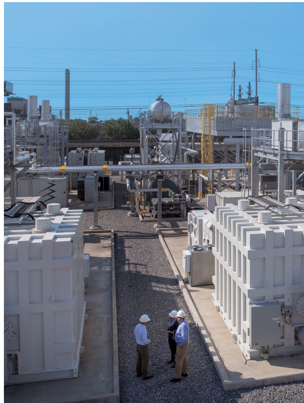
→ FuelCell Energy reports its 14.9MW fuel cell platform in Bridgeport, Connecticut, has provided clean and reliable power since 2013.
