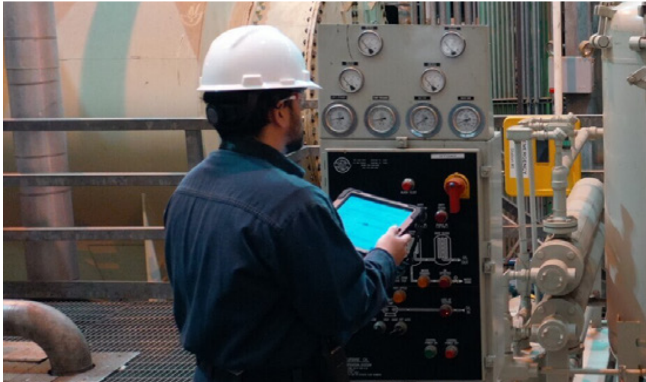
Remote Monitoring Center for Almerai, one of Saudi Arabia's largest food and beverage producers, uses APM from GE Digital to monitor the health of their equipment.
