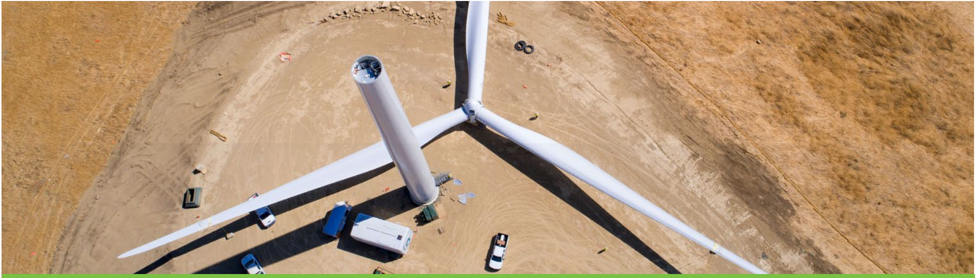
Construction of a wind turbine at NextEra Energy Resources' Golden Hills North Wind Energy Center in Livermore, California.
