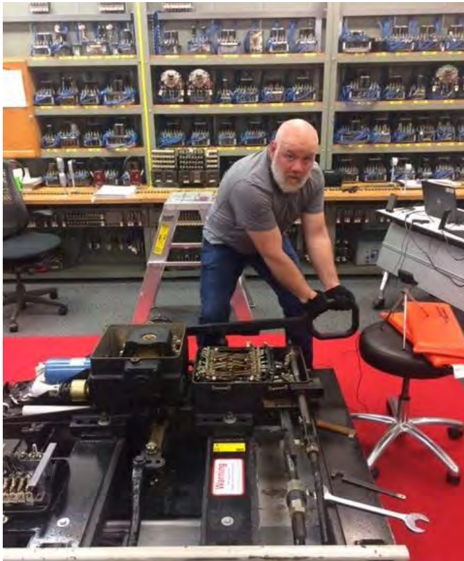
Joe Geis, senior instructor-Technical Training, Workforce Resources, demonstrates proper switch tension during a presentation at the Lone Star Training Center Signal Lab.
