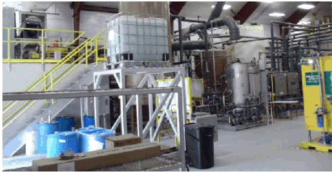
Union Pacific's new industrial wastewater treatment plant (IWTP) at the East Portal.
